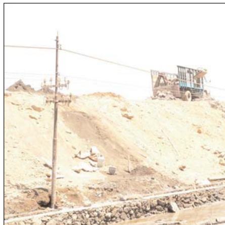
Dyke built in attempt to contain the mud. (DTE)
